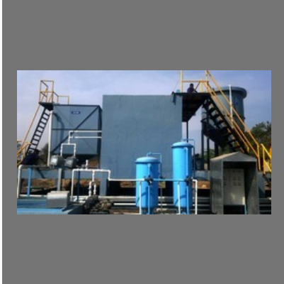
Effluent Treatment Plant
