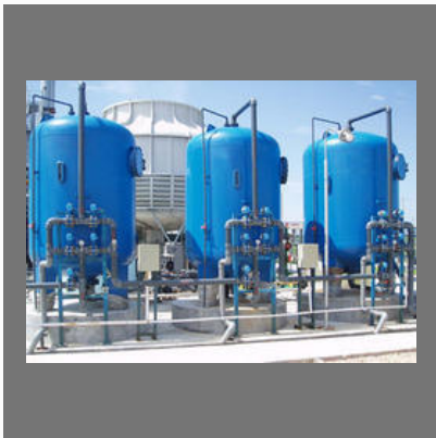
Iron Removal Plant
