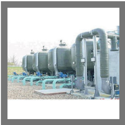
Compact Water Treatment Plant
