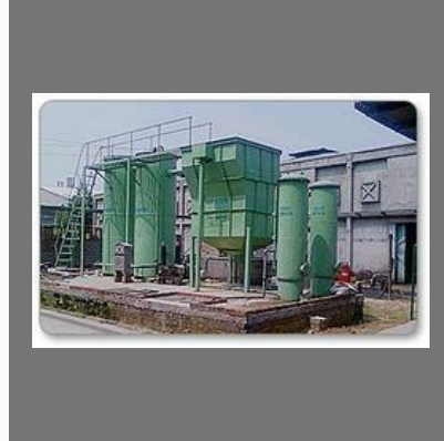
Industrial Sewage Treatment Plant
