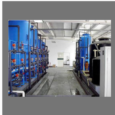
Industrial Water Softener
