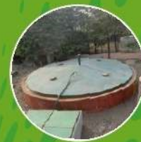
BIO GAS PLANT
